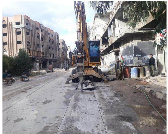
Road digger carrying out small-scale works on Yarmuk St. inside central Yarmuk camp earlier this year, at a time when many former residents of Yarmuk were speculating about the imminent release of reconstruction plans. Released on social media, early 2020.
