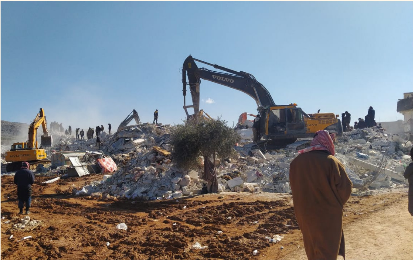
Earthquake response , Bseniah village, northwest Syria. Source: Mercy Corps, 2023.
