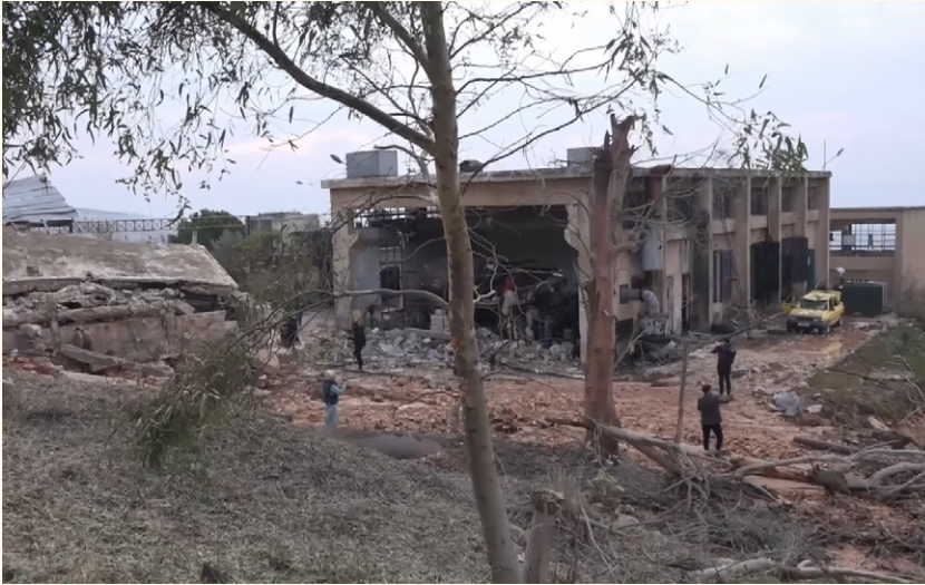
Image 4: The Al Arshani water station, west of Idleb City, sustained damage in January 2022 after alleged Russian airstrikes. Source: Orient News
